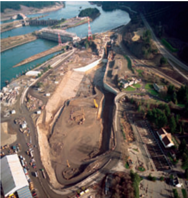
Using RCC application on the downstream guide wall decreased the construction time on the navigation lock. These photos show working on the tunnels for filling and emptying conduits and designing the concrete swing bridge.
