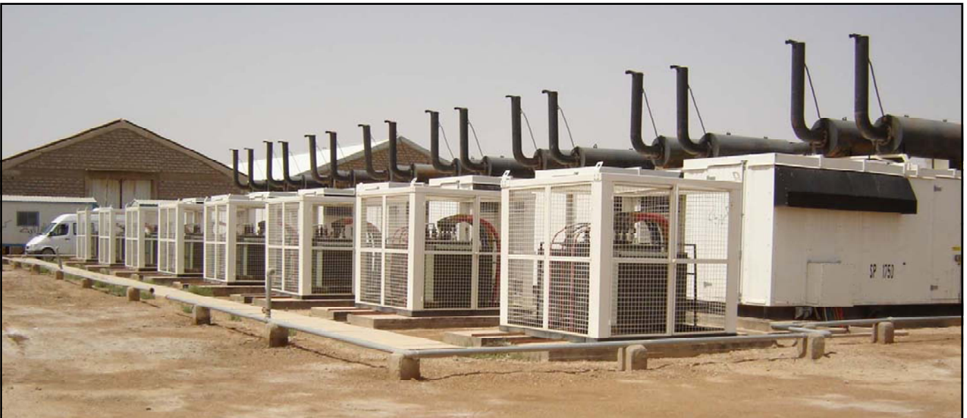
(Above) The Tameem Southeast generating facility will soon be fully operational providing 11 megawatts of additional electricity to the Ramadi grid in the Al Anbar Province of Iraq.
