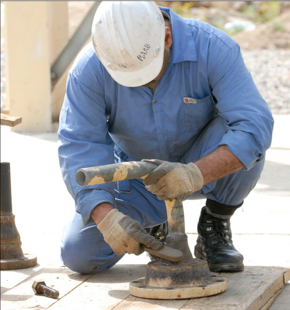
(Opposite page) Workers adjust settings on pipes at the South Rumaylah Central gas compressor station.
