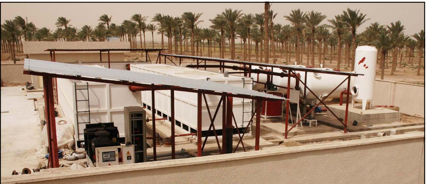
(Above) One of two water treatment facilities being managed by the Gulf Region Central district, U.S. Army Corps of Engineers, to bring improved water services to the residents in and around Ramadi, Iraq.
