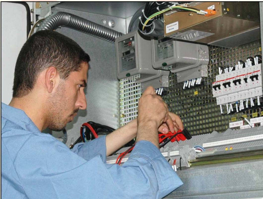
An Iraqi worker tests one of two new 33kV substations recently built in Fallujah to upgrade the city's electrical distribution network.
