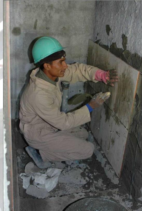
A skilled Iraqi craftsman installs ceramic tiles in a bathroom for a medical treatment facility at the site of the Nasiriyah Maximum Security Correctional Facility.
