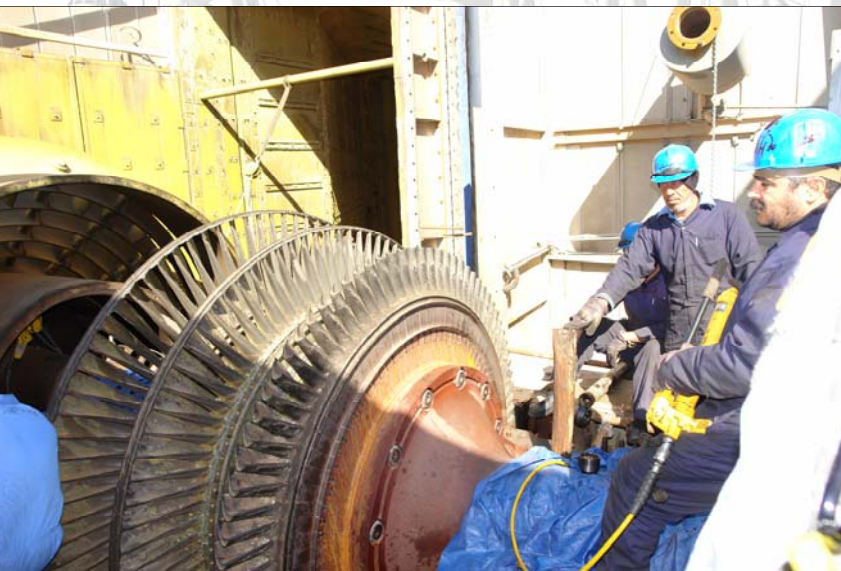
Iraqi workers repair one of the restored turbines at the Qudas plant.
