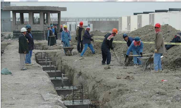
Iraqi construction workers prepare to refill a trench where concrete and re-bar footers have been recently installed. The new prison project employs an average of 200 workers a day, helping the local An Nasiriyah economy.
