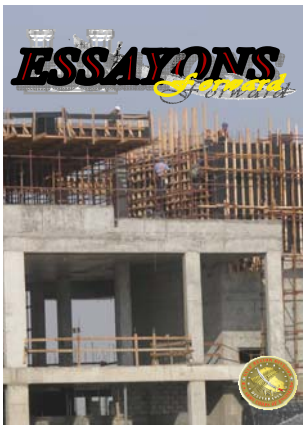
COVER: Work continues on the Basrah Children's Hospital in southern Iraq. (Photo by Thomas O'Hara)
