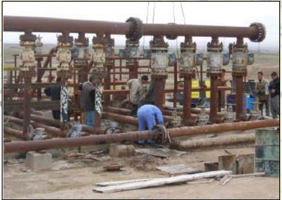
Construction was completed on three Gas and Oil Separation Plant projects in Basrah Province, totaling $15 million. The projects will help increase Iraq’s crude oil processing capacity, feed gas required to support liquid petroleum gas, and sustain crude oil flow in pipelines. (USACE photo)
