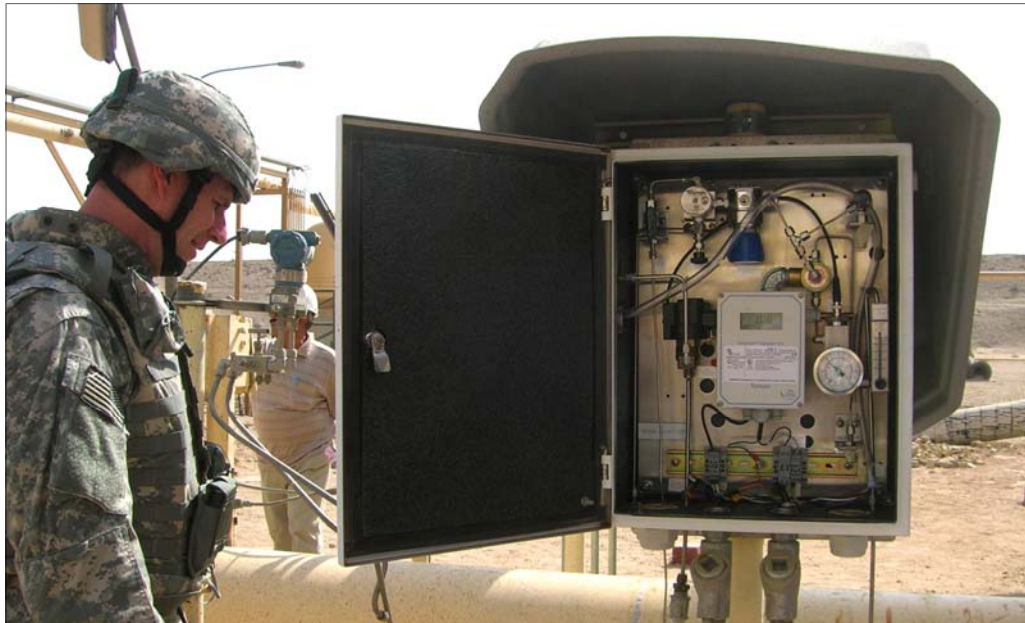
Sgt. 1st Class David Adland with the U.S. Army Corps of Engineers checks the construction and installation of an in-line moisture analyzer at Gas Compression Station 2 near the North Rumaylah Natural Gas Liquid (NGL) plant in the Al Basrah Province, Iraq. (Army photo)
