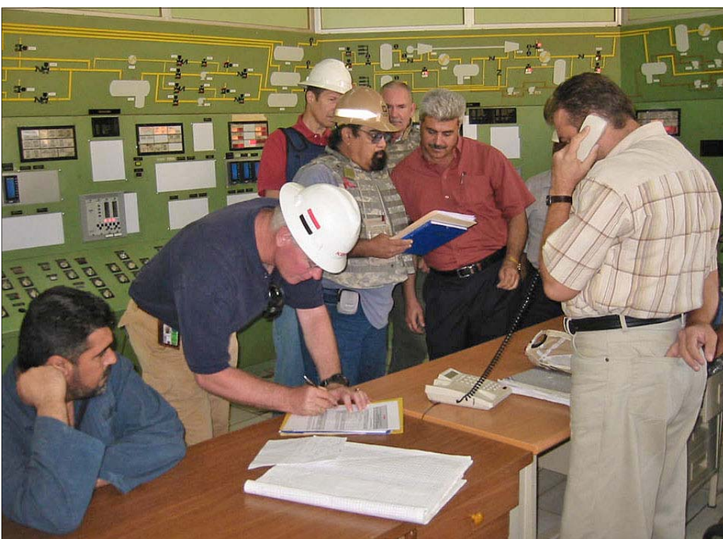
U.S. Army Corps of Engineers representative Ray Gonzales, center with beard, completes the project completion paperwork with the contractor and Southern Oil Company members at Compressor Station 5 in Rumaylah, Iraq. (Army photo)
