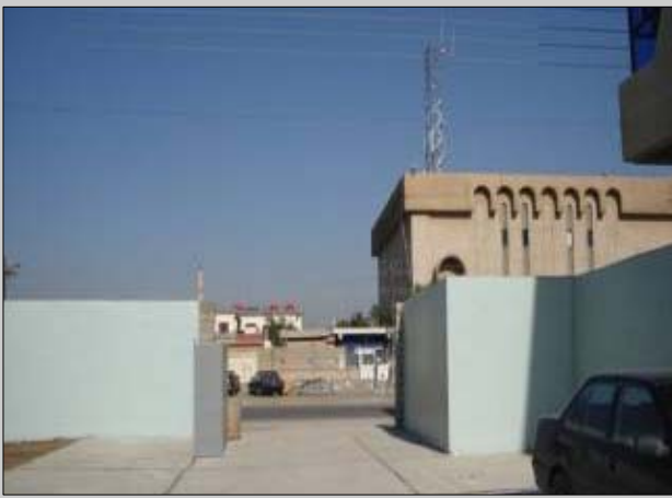
Saydea Fire Station Paving and security fencing project – Baghdad Province – completed Nov. 23
