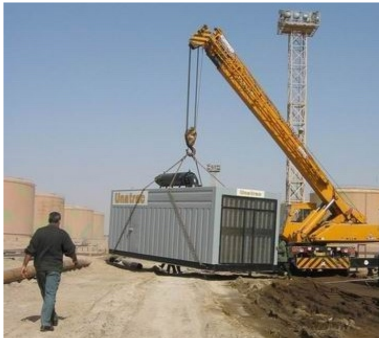
The Latifiyah fuel depot and distribution center, where power outages have led to fuel shortages, has more dependable power this week, arranged through the RIO directorate. This 1,000 KVA generator was purchased through the Coalition Provisional Authority using a portion of funds seized from the former regime. The depot serves about half of Baghdad's service stations.
