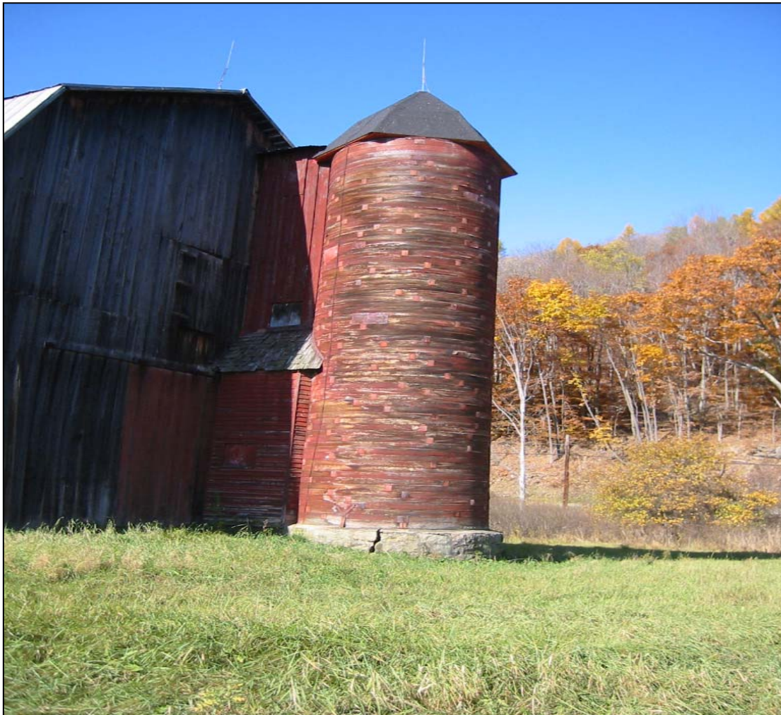
105-EU-001-15. Silo looking NW. This Potter County silo had its patent recorded on a sign affixed to the silo. First patented 1903, later revisions 1914 and 1915.
