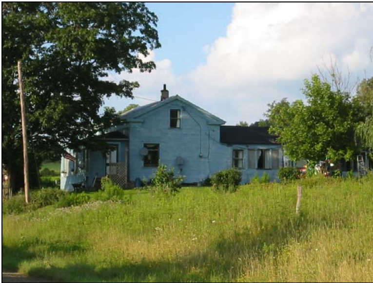
117-BR-001-04. S. Side of House, Tioga County. This house shows a more modest one and a half story variation on the theme.
