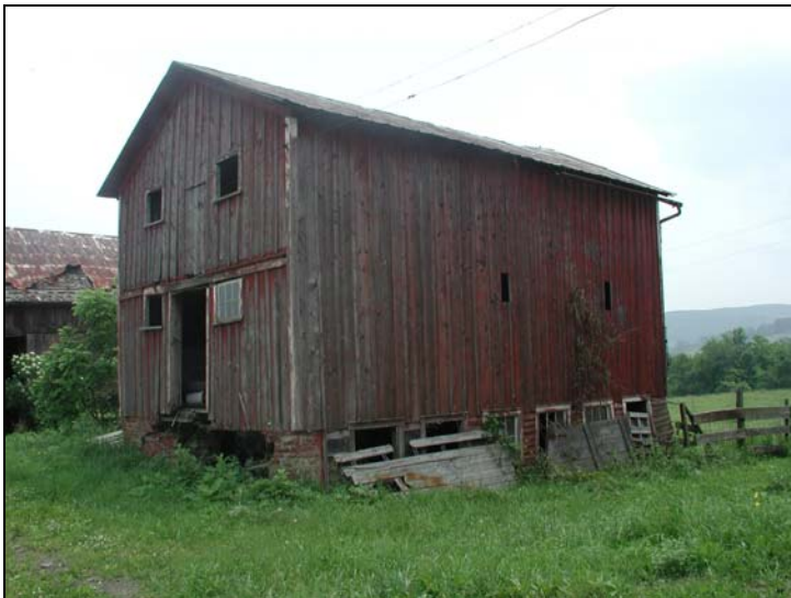
Bradford County, Josephus Campbell site. The blank wall, pass door, gable end openings, raised foundation, and interior partitions suggest that the upper part of this building may have been a granary.
