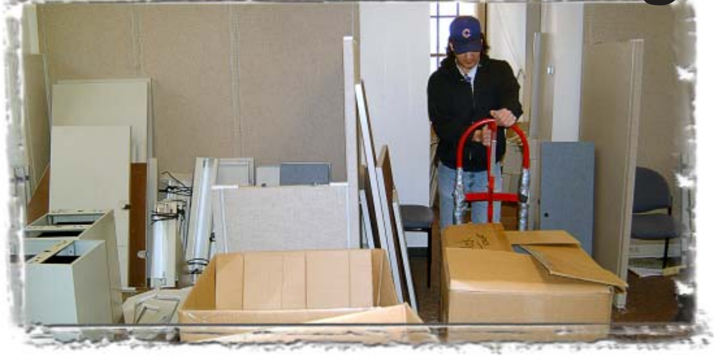
Left - Ceiling tiles and other debris float on top of standing water inside the Natural Resources Management section of Operations Division on the third floor of the Clock Tower Building. This area was directly affected by the leak because it sits below the area where the water pipe burst. Photo by Angela Rursch, Information Management. Above - An employee contracted from Saxton Inc, a Davenport, Iowa, facilities management company, boxes up cubicle parts for storage while the water-damaged spaces are renovated. Photo by Mark Kane.
