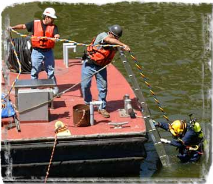
Above - Al St. Clair, Mississippi River Maintenance Crew, slowly submerges into the water inside the lock chamber before checking a key area of the lock wall for any possible obstacles, while (from left to right) Ron Wunderle and Charlie Lovell, Mississippi River Maintenance Crew, make sure his line doesn't get hung up.
