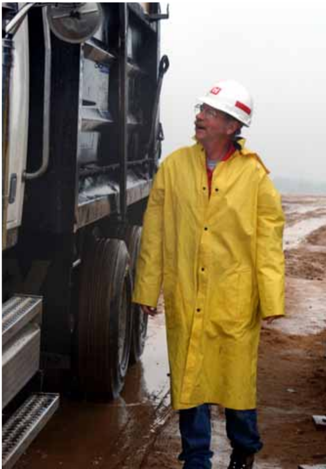
Left - Lee Schweiger, Construction Division, checks in a truck delivering debris to a reduction site during Hurricane Ivan Relief Operations in South Alabama. Photo by Tim White, U.S. Army Engineering and Support Center, Public Affairs.
