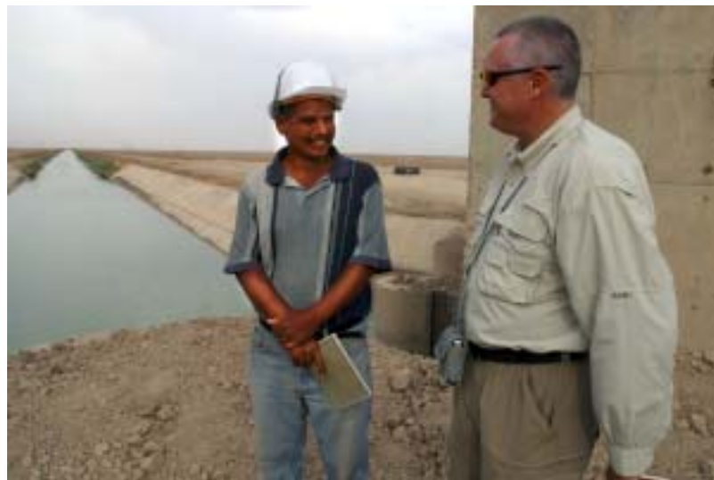
Corps project manager for the Sweet Water Canal Project, Chuck VanLaarhoven, and Iraqi site engineer, Abdul Karim Ali, inspect ongoing work at the canal. Photo by Thomas Hartwell, USAID contract photographer, www.usaid.gov .
