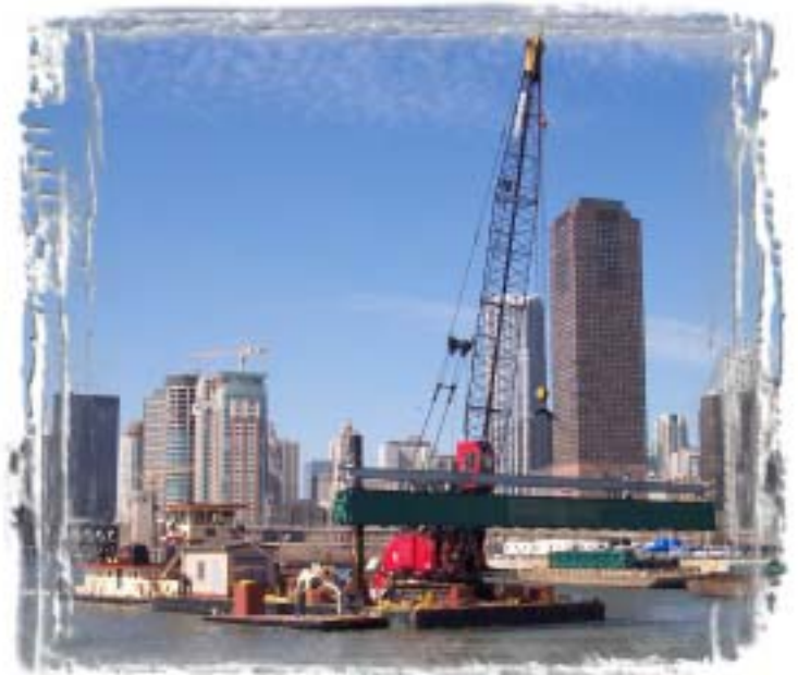
The crew of the MV Creve Coeur use the Manitowac 3900 crane to lift a bulkhead section during the team’s work at the Chicago Lock.
