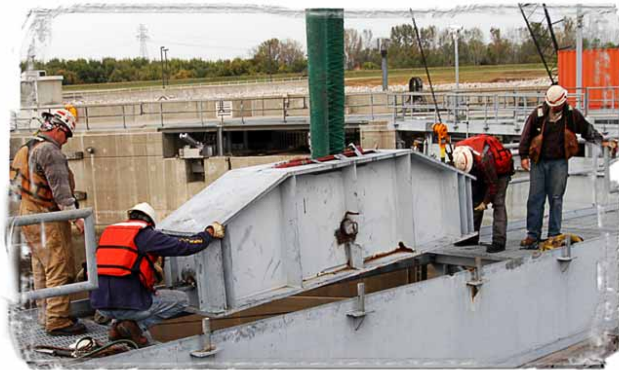
The Strongback is lowered into place on the Missouri gate with the help of Bryon Ray, Doug Schaer, Brian Smith, and Doug Morgan, Illinois Waterway Project Office Maintenance Unit 1.
