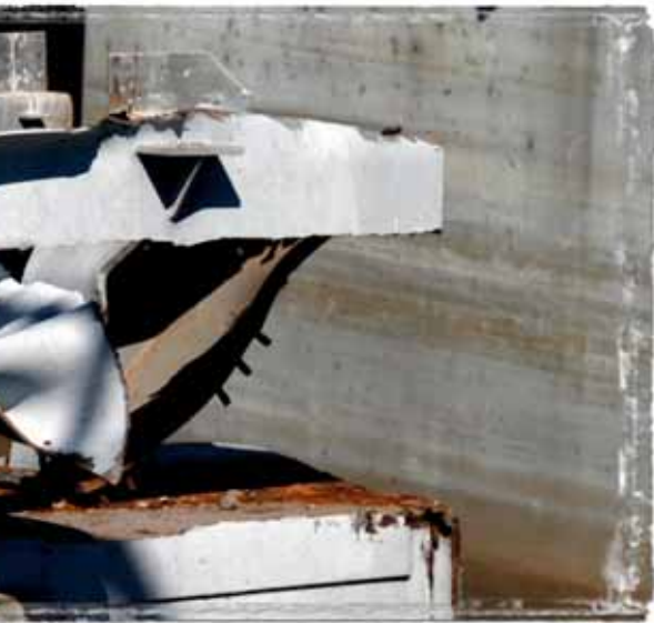
A closer view of the damage caused to the Missouri gate at the Mel Price Auxiliary Lock.
