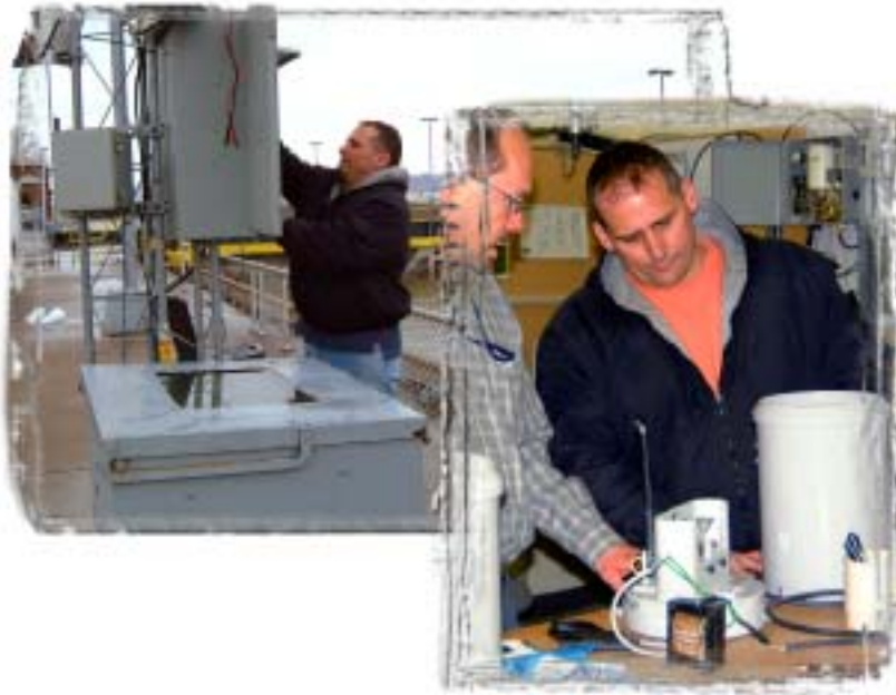
(Left photo) VanWatermeulen works with weather equipment at Locks and Dam 14 and (right photo) at District headquarters with Jim Stiman (left), Engineering Division.
