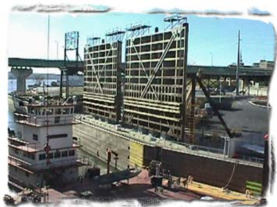
The original lower miter gates, resting in supports, loom over Lock 19 after being removed from the lock for the first time since 1957. The Motor Vessel Bettendorf is seen to the left. Photo by Gene Walters, assistant lockmaster, Lock and Dam 19.
