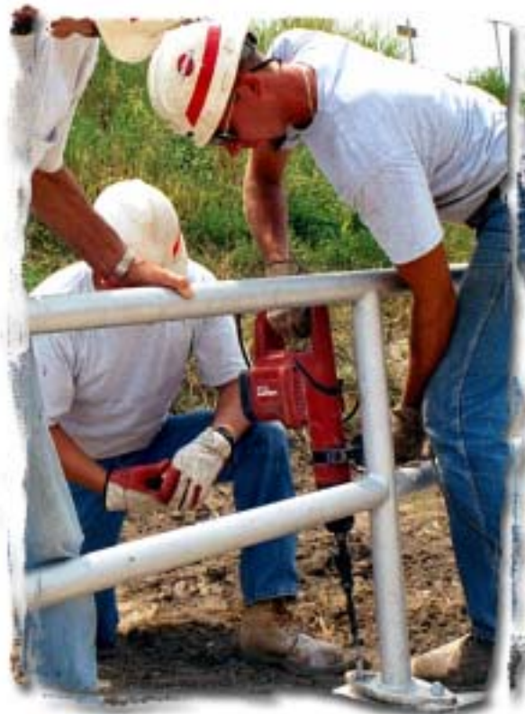
Jared Miller operates a Hammer drill during a handrail installation project at Dresden Island Lock and Dam. Also pictured is Russell Stilwell (left) and Ed Picken (center), both from Illinois Waterway Maintenance Structures Unit 2.
