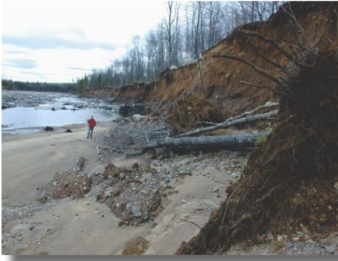
Before EWP recovery assistance: Severe streambank erosion downstream of the basin. (May 2003)
