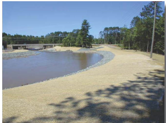
After EWP recovery assistance: Tourist Park stream banks were reshaped, seeded, and stabilized with rock rip-rap. (July 2003)
