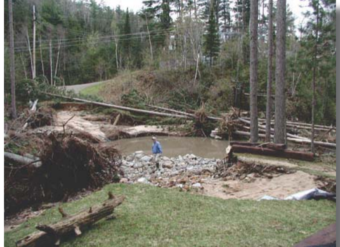
Road washout after the flood.
