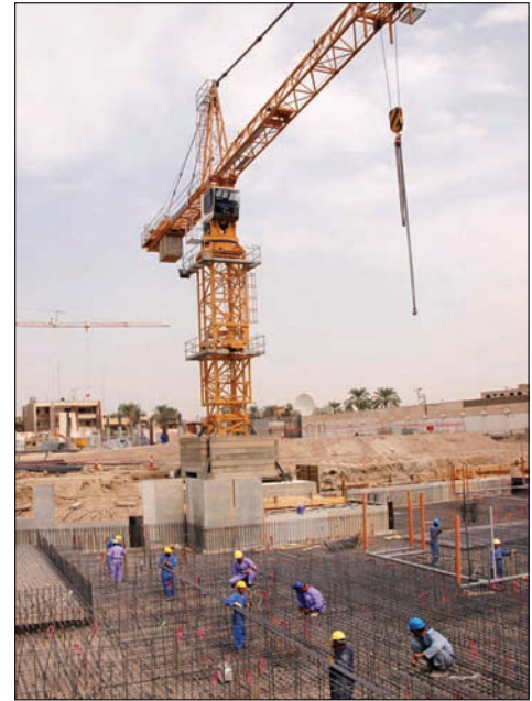
Work continues at the $22.7 million Al Mamoon Exchange and Telecommunications facility in Baghdad.
