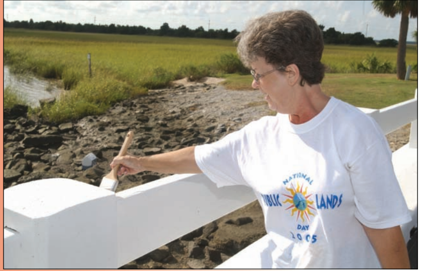
Patricia Gibbs, a procurement technician with the district lends a hand at Fort Pulaski National Monument by painting a bridge in observance of National Public Lands Day on Sept. 24.
