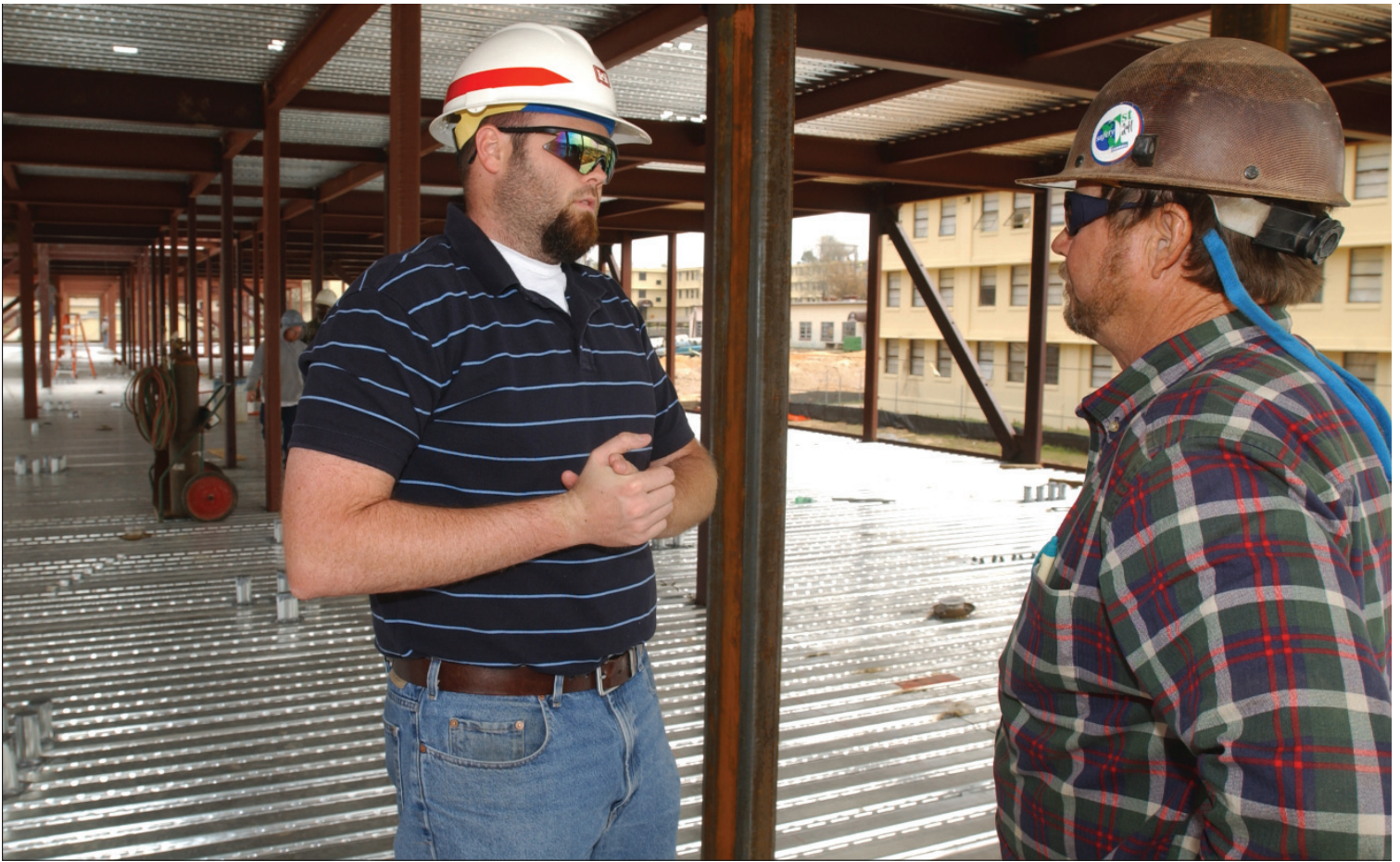
Photo (Above): Chad McCloud, civil engineer and a contractor representative discuss construction of the new Kelly Hill barracks at Ft. Benning. (Below): Leroy, Fedd, construction representative, inspects the exhaust venting for the fire engines at the new firestation. The new one-story firestation, which replaces the old firestation built in 1937, comes complete with a kitchen, dayroom, sleeping quarters, administrative offices, a medical room, and an apparatus storage room.
