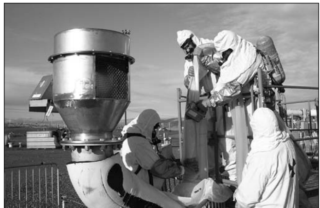
Workers retrieve cameras used in tank C-108 retrieval. Tank C-108 is the ninth Hanford single shell tank to be in retrieval or completed
