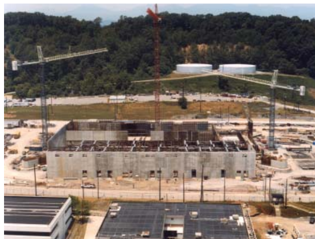
View of the Highly Enriched Uranium Materials Facility Under Construction at Y-12
