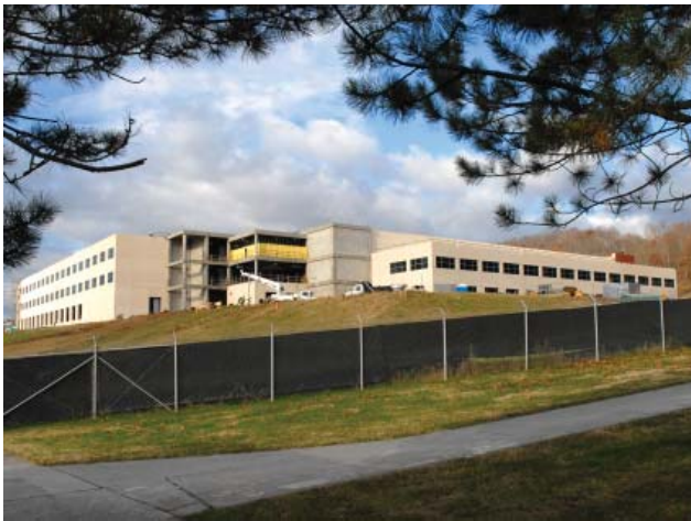
View of the Privately Financed Jack Case Center Under Construction at Y-12
