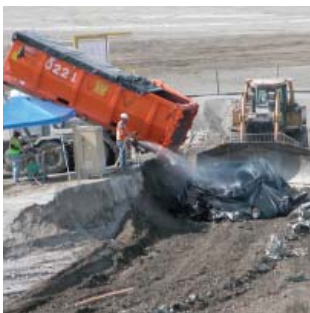
Contaminated Soil and Other Material from Hanford's River Corridor Is Being Disposed of in the Environmental Restoration Disposal Facility. Water Is Being Applied for Dust Control
