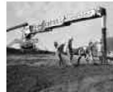
WORKERS FINISH CONCRETE POURS AT THE Y-12 HIGHLY ENRICHED URANIUM MATERIALS FACILITY PRESENTLY UNDER CONSTRUCTION.
