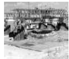
TWO OF FERNALD'S MOST RECOGNIZABLE LANDMARKS FELL TO THE GROUND ON APRIL 16-17, 2005.
