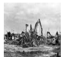
THE B444 WAS THE PRIMARY NON-NUCLEAR MANUFACTURING FACILITY AT ROCKY FLATS. THIS IS THE LAST OF FOUR ORIGINAL PRODUCTION FACILITIES BUILT IN THE EARLY 1950'S TO BE DEMOLISHED.
