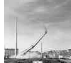
DEMOLITION EXPERTS DETONATED CHARGES TO COLLAPSE A 250 FT. EXHAUST STACK AT THE TEST REACTOR AREA.
