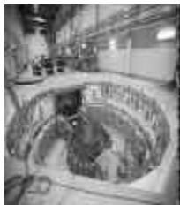
CONSTRUCTION IN THE INTERIOR OF THE SPALLATION NEUTRON SOURCE AT THE OAK RIDGE NATIONAL LABORATORY.
