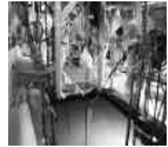
DEBRIS REMOVAL FROM THE K-EAST BASIN REQUIRES FULL RADIATION PROTECTION CLOTHING AND AIR PURIFYING RESPIRATORS.
