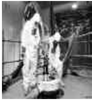
WORKERS USING PNEUMATIC AND MECHANICAL RETRIEVAL SYSTEMS TO REMOVE WASTE FROM THE SILO AND PACKAGE IT IN SOFT-SIDED CONTAINERS FOR OFF-SITE SHIPMENT.
