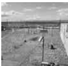
ANCILLARY FACILITIES NEAR U PLANT
