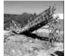
THE DECONTAMINATION AND DEMOLITION PROJECT WORKS SCOPE INCLUDES THE DISMANTLEMENT OF 259 FORMER PRODUCTION PLANTS, SUPPORT STRUCTURES AND ASSOCIATED COMPONENTS.
