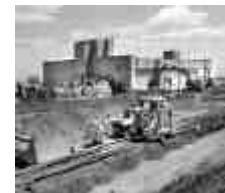
WORK TO INSTALL A RAIL LINE FOR SHIPPING B371 BUILDING RUBBLE. THE PROJECT NEARS COMPLETION AS PHASE III DEMOLITION BEGINS.
