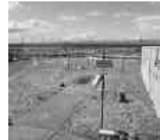
THE HOSE-IN-HOSE SYSTEM AT K-EAST BASIN.
