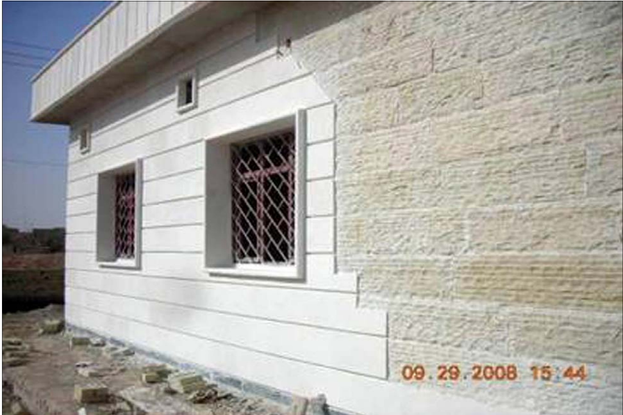
Iraqi workers are building the $500,000 Al Jumhoury new primary healthcare clinic in Diwaniyah, Qudisiyah Province, southern Iraq [USACE Photo]
