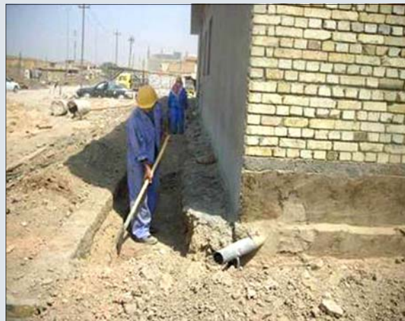
Iraqi workers are building the $500,000 Al Jumhoury new primary healthcare clinic in Diwaniyah, Qudisiyah Province, southern Iraq [USACE Photo]
