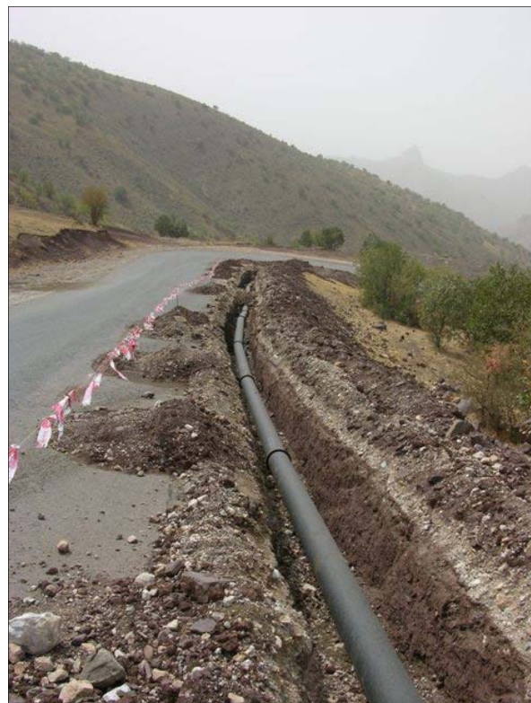
Five miles of pipe delivers mountaintop spring water to the town of Choman below and its two neighboring villages, where it connects to an existing water network [USACE Photo by LuAnne Fantasia]
