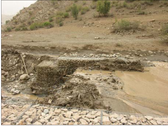
Phase II of the Rosti Valley project is currently ongoing and will prevent future damage to the agriculture and irrigation for the people of the valley's 17 villages. A 23-foot-high gabion weir toward the top of the mountain provides most of the protection, breaking initial current of flood waters. There are 15 other locations down river, each with a series of 10-foot-high gabions, as seen in this photo. [USACE Photo by LuAnne Fantasia]
