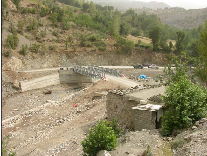
Rosti Valley Phase I bridge: During Phase I of the Rosti Valley project, a bridge was replaced that was critical for passage to 17 villages up and down the mountain river. This project also included the massive cleanup of debris from a flash flood in the spring of 2007. [USACE Photo by LuAnne Fantasia]
