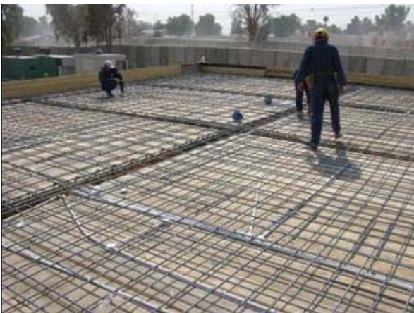
Electrical conduits are installed and Iraqi workers are ready to place the concrete roof on the new enlisted Soldiers' barracks of the Ninewa Operations Center. When Phase II is finished in mid-November, General Riyadh and his command and staff will have a new kitchen and dining areas, as well. [USACE Photo by LuAnne Fantasia]
