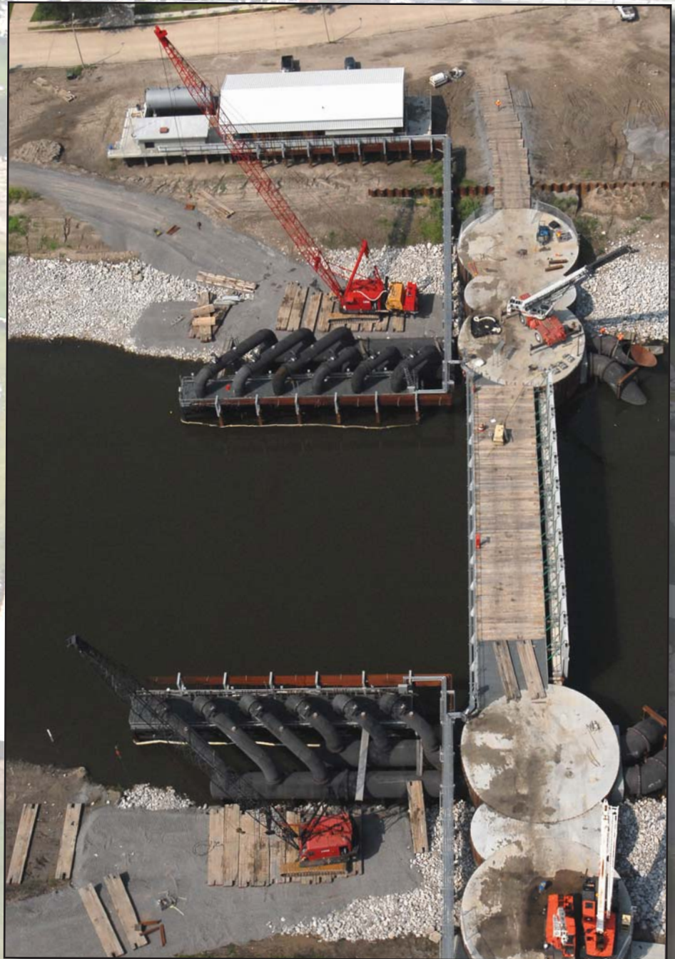
An aerial view of the London Ave. Canal with its platforms and new temporary pumps. (USACE Photo)
