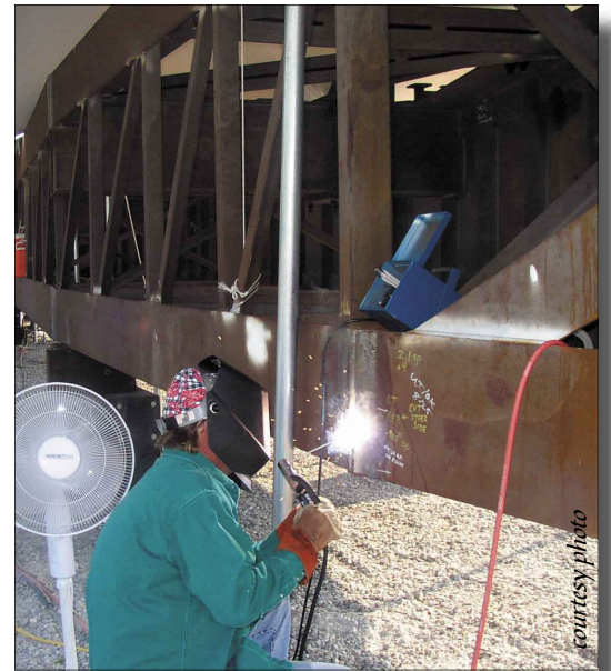
Small business Southern Services & Equipment Inc. repairs a stop log at Port Allen Lock, a $1.6 million job.
