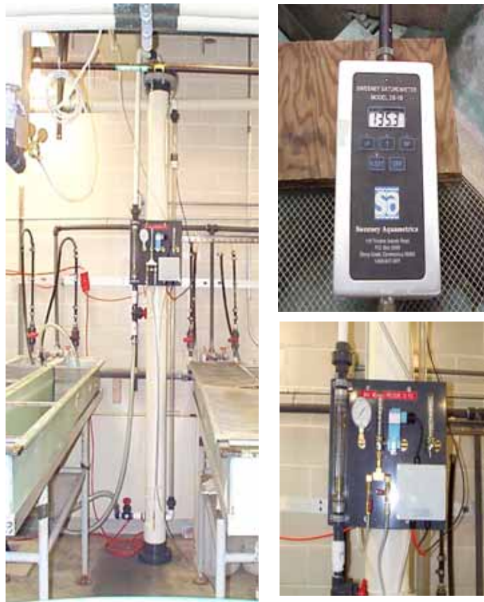
Figure 2.3. Gas-supersaturation system showing controls (lower right) and saturometer (upper right).
