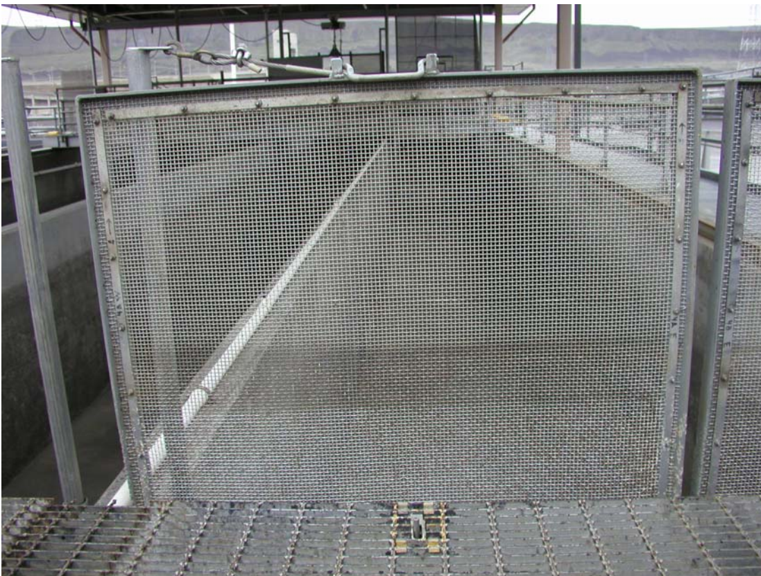
Figure 7. Raceway exit screen at juvenile bypass system.
