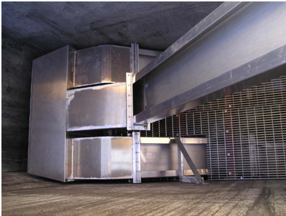
Figure 6. View from above of the Washington-shore AWS LPS collector ramps, and first rest box.
