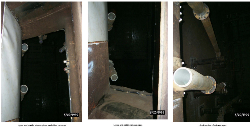
Figure A - 12. Photos of McNary fish release piping at stay vane
