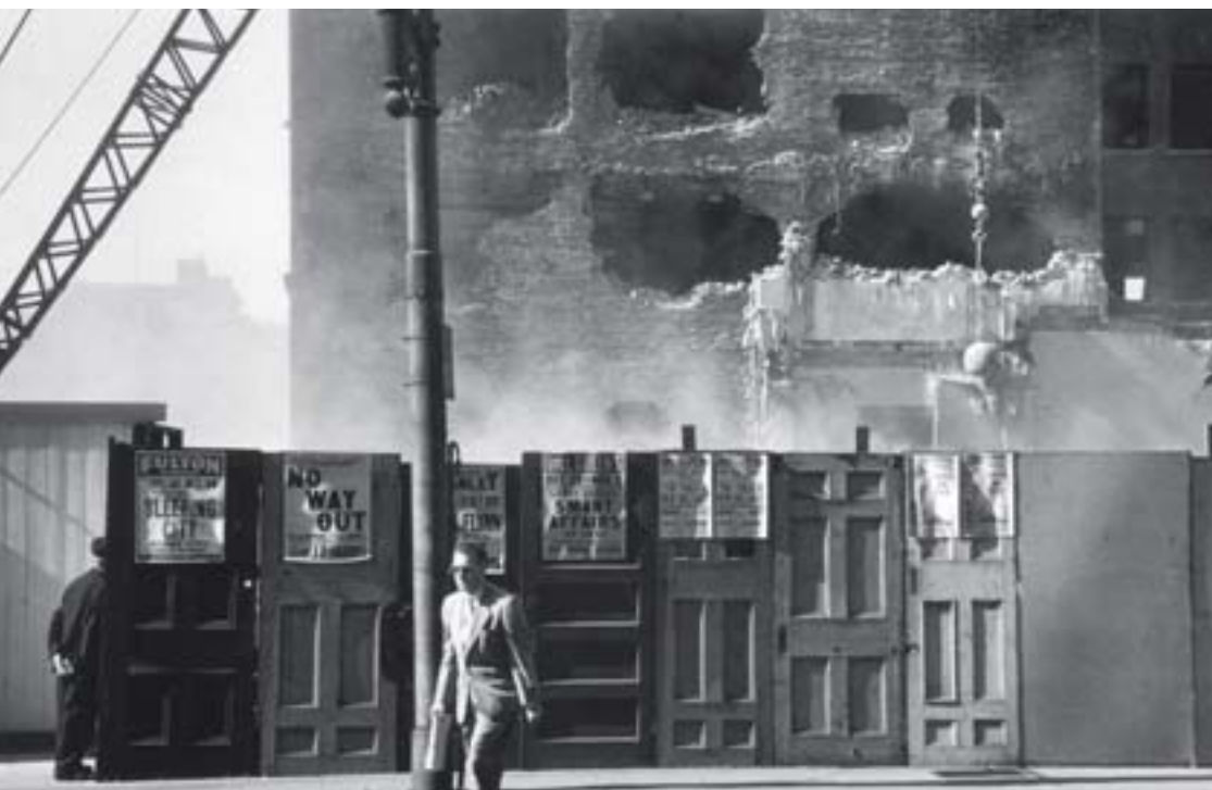
Gateway Center Demolition Area. Elliott Erwitt. October 1950. “Many of [Erwitt’s] best Pittsburgh photographs present the viewer with powerful contradictions,” say Schulz and Plattner.
