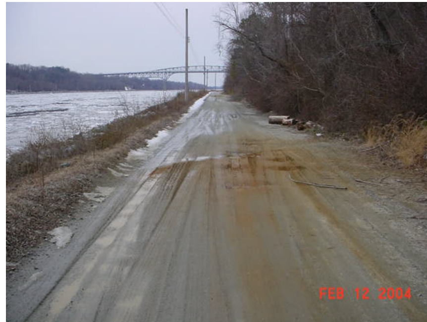
PHOTO 4. STATION 51+250, NORTH SIDE, LOOKING WEST, 12 FEB 04. EAST FLANK OF SLOPE FAILURE.
