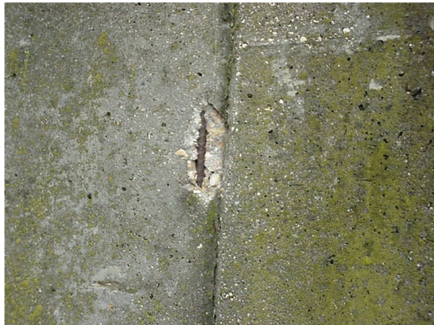
PHOTO 3. STATION 29+250, SOUTH SIDE, 30 AUG 04. SPALL WITH REBAR SHOWING IN THE RETAINING WALL SHOWN IN PHOTO 2.
