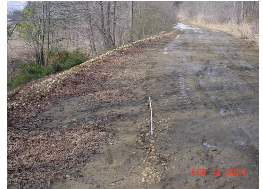
PHOTO 6. STATION 54+900, NORTH SIDE, LOOKING WEST, 12 FEB 04. CRACKING ALONG EDGE OF SECOND LEVEL ROAD.
