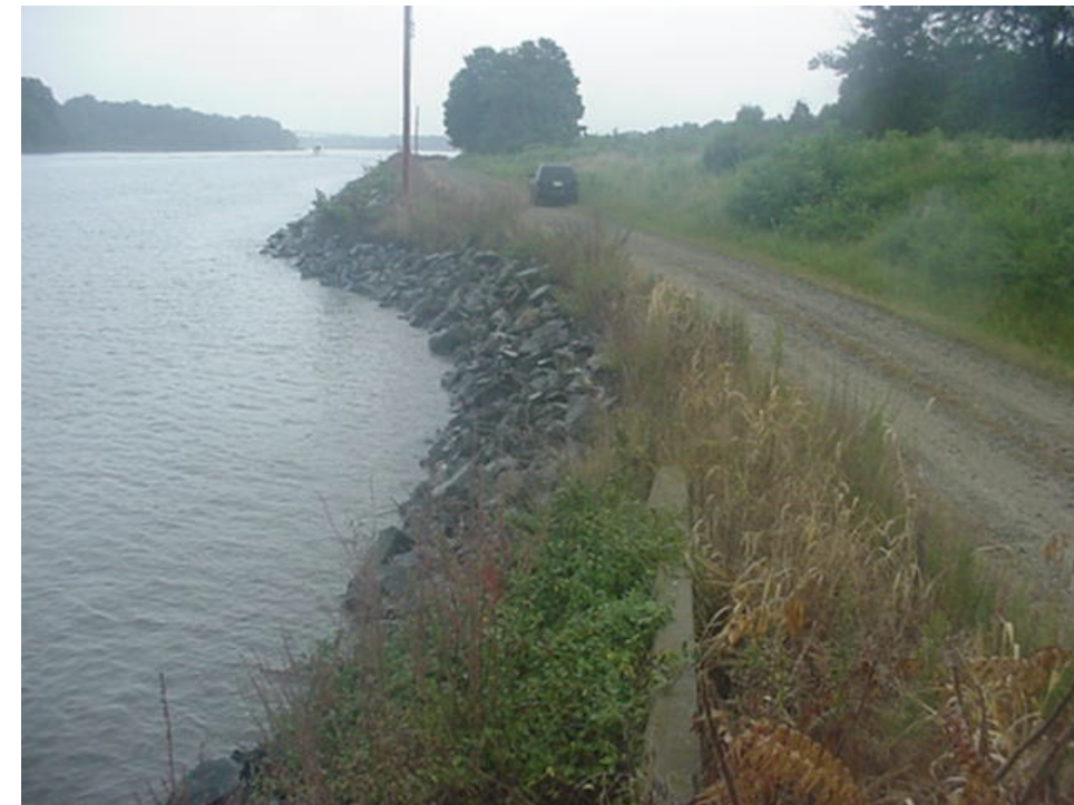
PHOTO 1. STATION 21+200, NORTH SIDE, LOOKING WEST, 30 AUG 04. LOCATION OF A PREVIOUS SLOPE FAILURE. THIS AREA WAS CUT BACK AND PROTECTED WITH RIPRAP.
