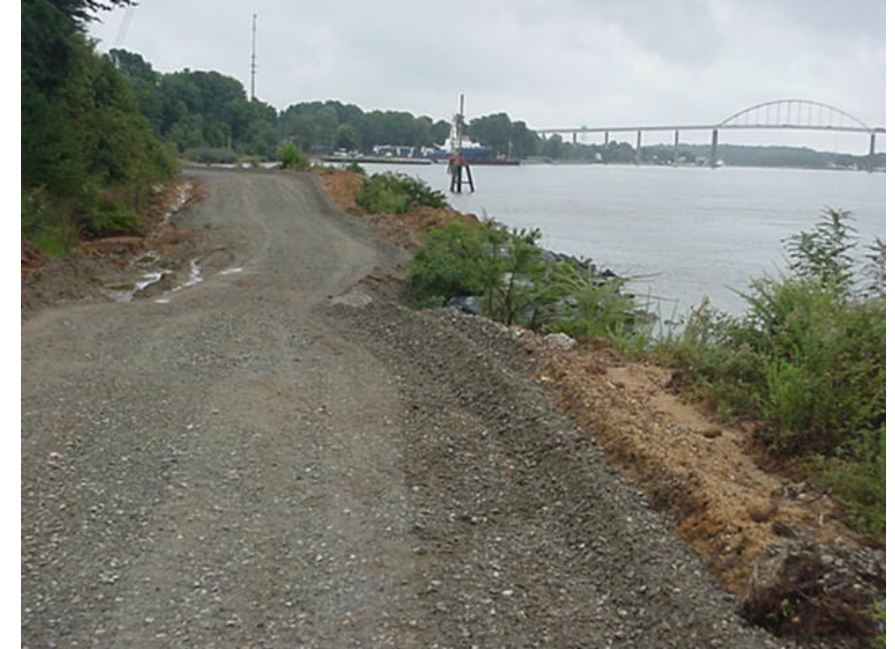
PHOTO 13. STATION 58+500, NORTH SIDE, LOOKING EAST, 30 AUG 04. WEST FLANK OF SLOPE FAILURE.
