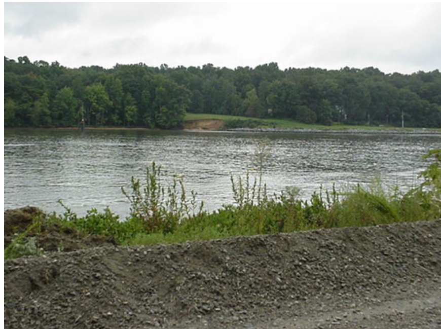
PHOTO 15. STATION 84+000, SOUTH SIDE, 30 AUG 04. LOOKING AT THE SLOUGHING FROM THE NORTH SIDE OF THE CANAL.
