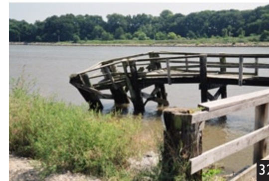
DAMAGED ST. GEORGES FISHING PIER
