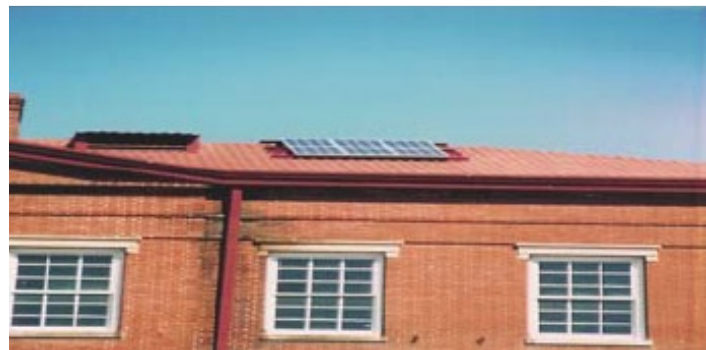
SOLAR ROOF PANELS ON FORT DELAWARE - COURTESY OF BIO-SUN
