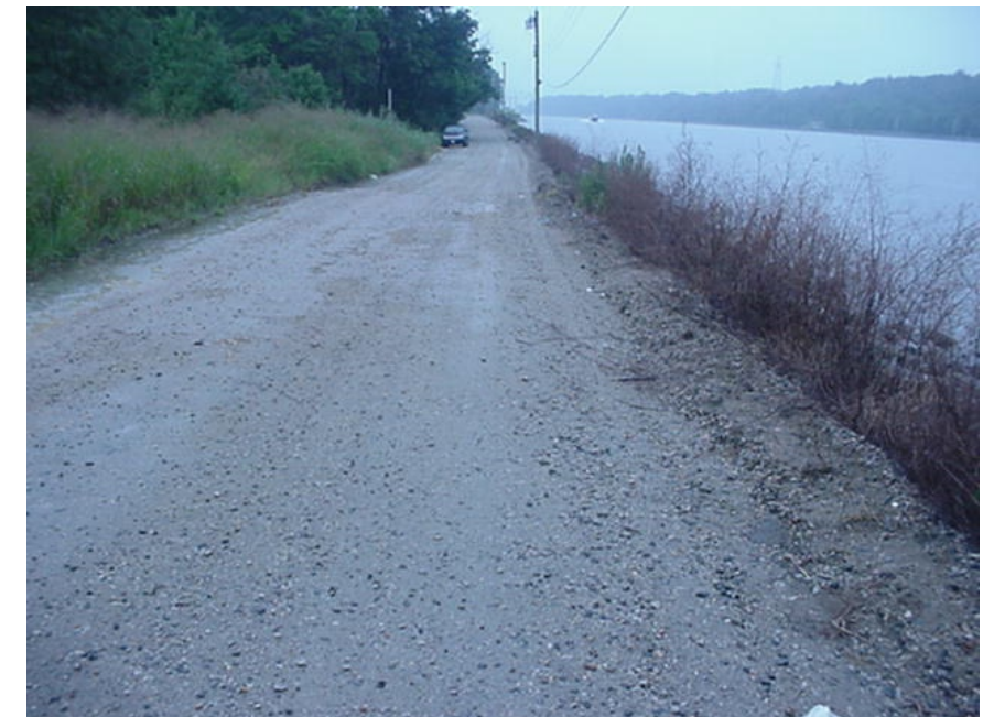
PHOTO 7. STATION 54+900, NORTH SIDE, LOOKING EAST, 30 AUG 04. WEST FLANK OF SLOPE FAILURE.
