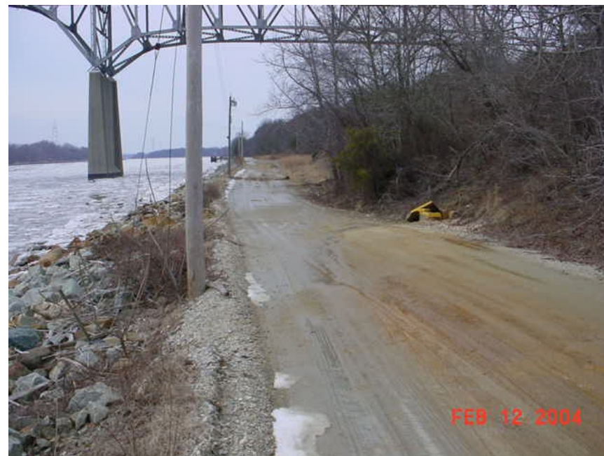
PHOTO 5. STATION 54+900, NORTH SIDE, LOOKING WEST, 12 FEB 04. EAST FLANK OF SLOPE FAILURE.
