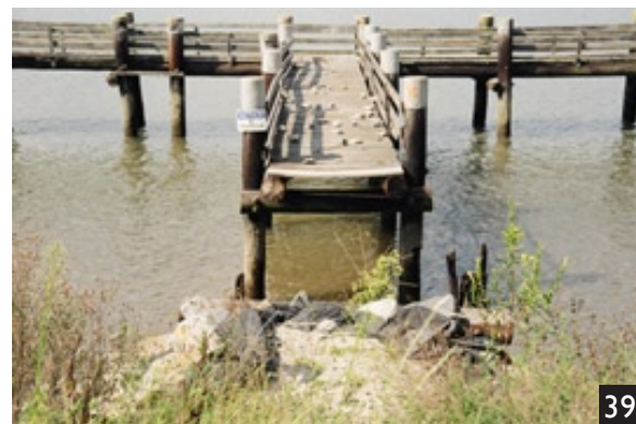
DAMAGED FISHING PIER WEST OF S.R. I BRIDGE
