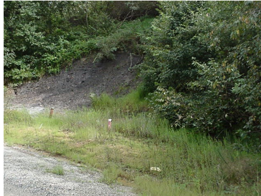
PHOTO 10. STATION 58+500, NORTH SIDE, 30 AUG 04. LOOKING ALONG THE WEST FLANK AT THE HEAD OF THE SLOPE FAILURE.
