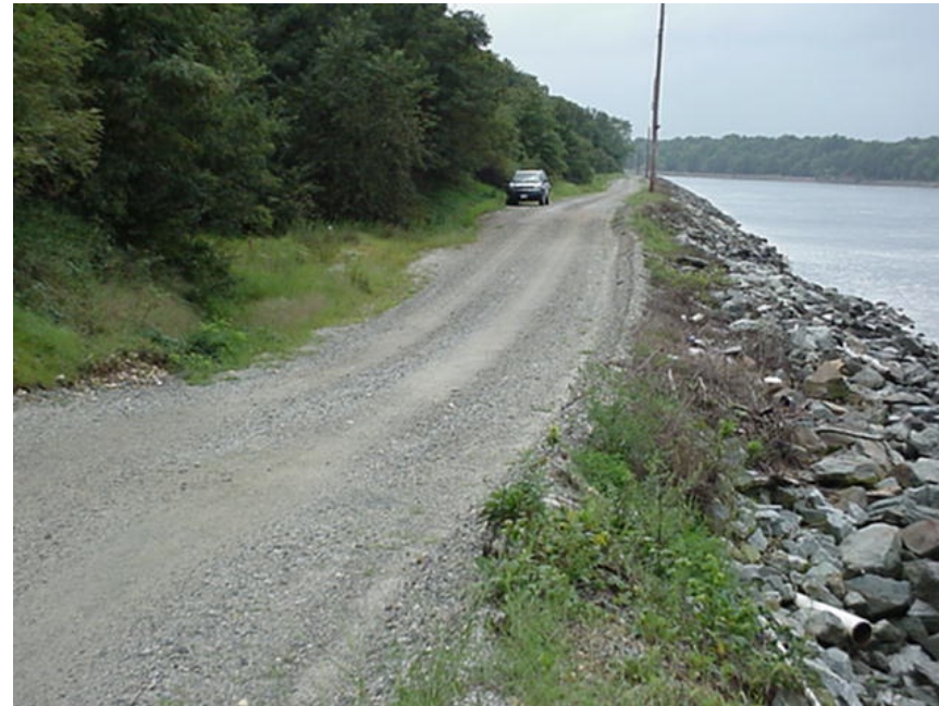
PHOTO 11. STATION 58+500, NORTH SIDE, LOOKING WEST, 30 AUG 04. EAST FLANK OF SLOPE FAILURE.
