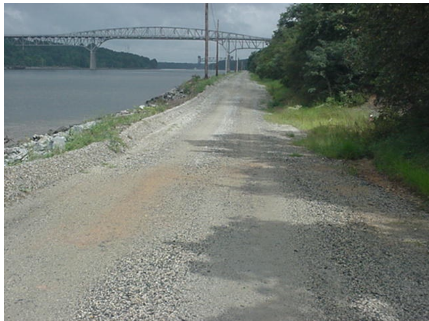
PHOTO 9. STATION 58+500, NORTH SIDE, LOOKING EAST, 30 AUG 04. WEST FLANK OF SLOPE FAILURE.
