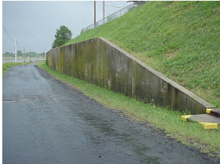
PHOTO 2. STATION 29+250, SOUTH SIDE, LOOKING EAST, 30 AUG 04. CONCRETE RETAINING WALL AT ST. GEORGES.
