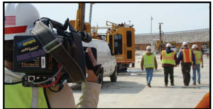
A cameraman films as Larry Craig (Wolf Creek Power Plant), Brook Brosi (Wolf Creek Resident Office), Mike Zoccola (Civil Design Branch), and Paul Ross (Wolf Creek Resident Office) walk the grouting work platform at Wolf Creek Dam.
