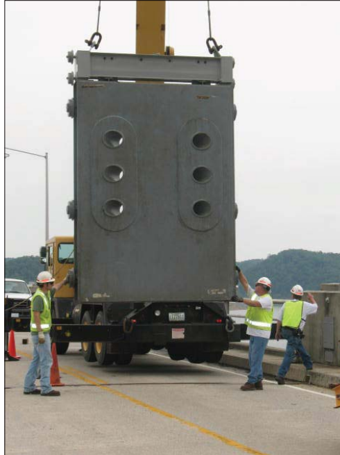
A crane hoists the orifice gate that was removed from Wolf Creek Dam.
