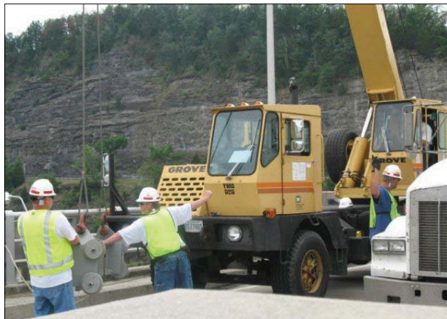
Chuck Ervin (Laurel) signals Brandon Masion-gale (Dale Hollow) in the crane, while John Roberson (Wolf Creek) steadies the auxiliary hoist and Christopher Marlow (Wolf Creek) directs large semis around the crane.
