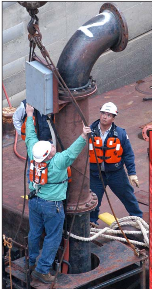
Bobby Holt (right) and Anthony Certeza rig a dewatering pump March 7 so it can be set in place by Derrick Boat Operator Jason Bradley (right inset) to pump the water from Cordell Hull Lock.
