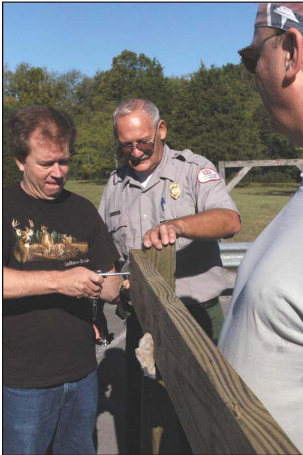
Corps Ranger Gary Conley assists two members of the Pine Creek Archery Club Sept. 18 in construction of a new target for the range. A total of 50 volunteers helped make NPLD at Old Hickory a success.
