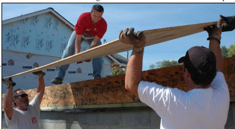
Butch Witcher (left) and Gary Davis lift flooring up to Kayl Kite on the Providence Park job site.
