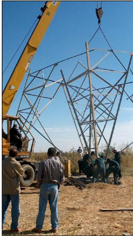
Workers erect one of the many towers that will carry electricity throughout the country of Iraq.
