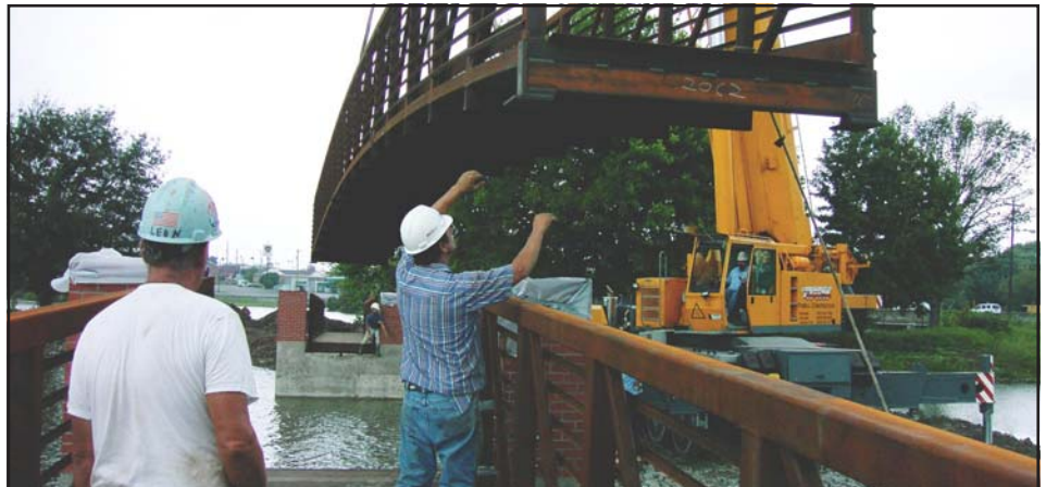
New Resident Engineer David Loyd captured this image of a bridge installation at the Drakes Creek Ecosystem Restoration Project in Hendersonville, Tenn.
