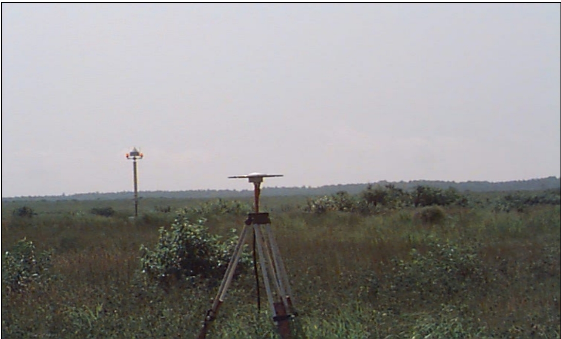
Figure 7: ACY LAAS IONO Station Antenna (with IMLA)
