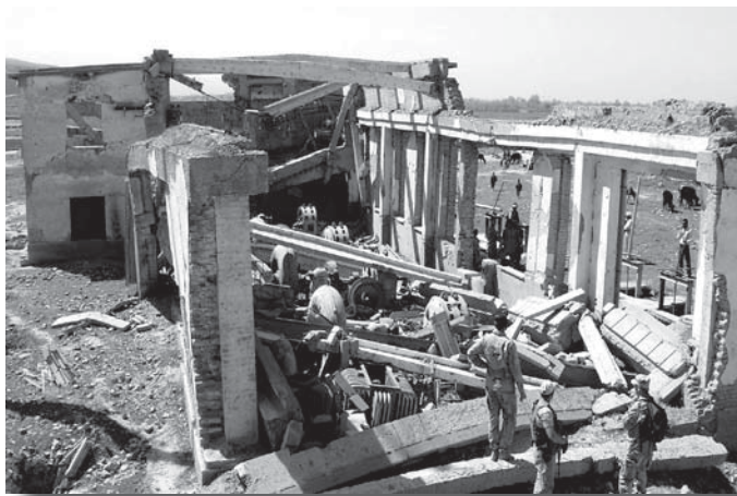
The Corps team inspects the severely damaged Khanabad power plant. The Taliban used the structure as a hideout after Sept. 11, 2001, before U.S. forces bombed it.
