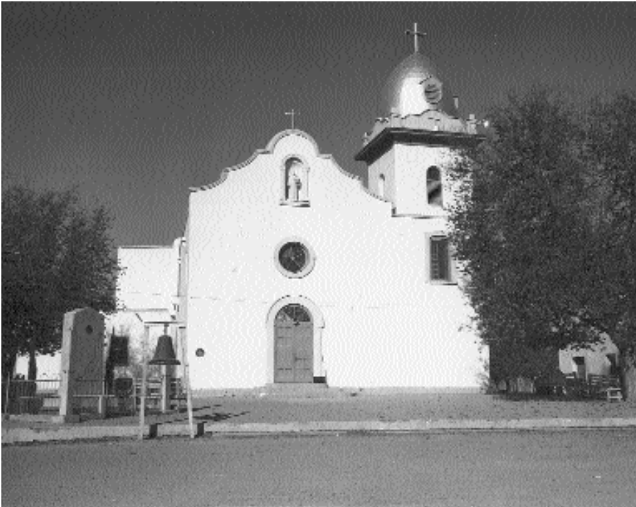
Work is presently underway to restore the Ysleta Mission, starting with the bell tower. Photo courtesy Texas Historical Commission.
