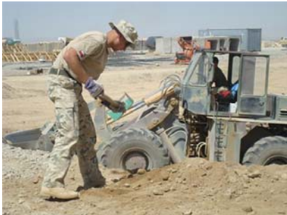
Polish Pvt. Piotr Oparski works on the final touches of a culvert as a scoop loader hauls the rest of the dirt.
