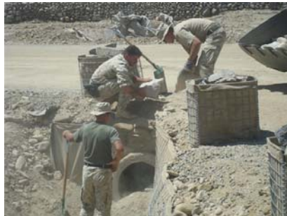
Korean soldiers work on a structure that will improve maintenance support for Forward Operating Base Sharana, Afghanistan.
