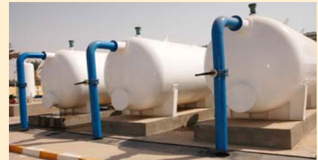
Iraq - The Shuhada Water Treatment Plant, located west of Fallujah, became fully operational and is producing enough drinking water to support the 10,000 residents in that area. (USACE Army Photo)
