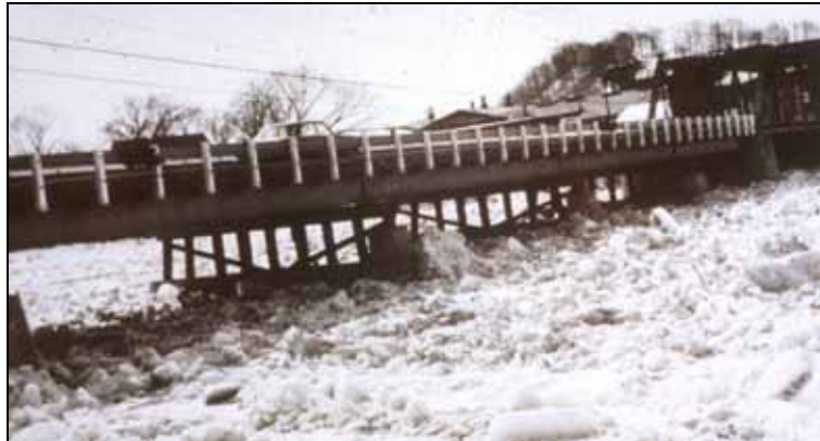
Figure 1. Temporary bridge piers subjected to ice forces in 1969.
