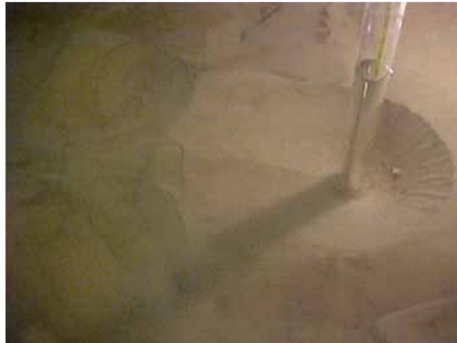
Figure A25. Final photo of scour hole; flow from right to left.
