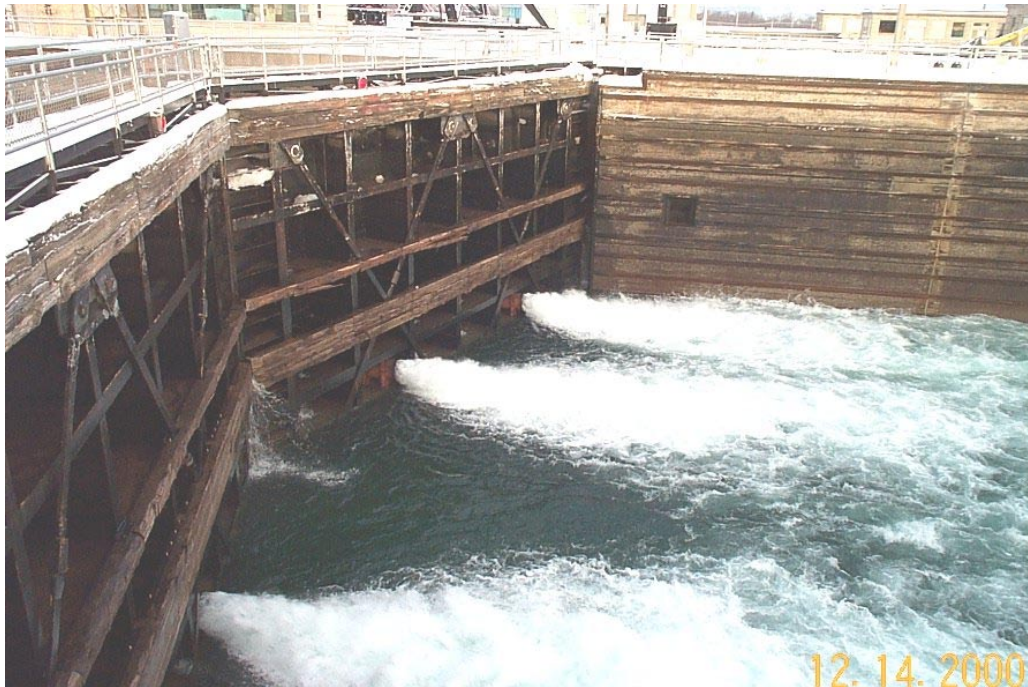
Figure 15. Ice flushing manifolds at the Poe Lock, Sault Ste. Marie, Michigan.
