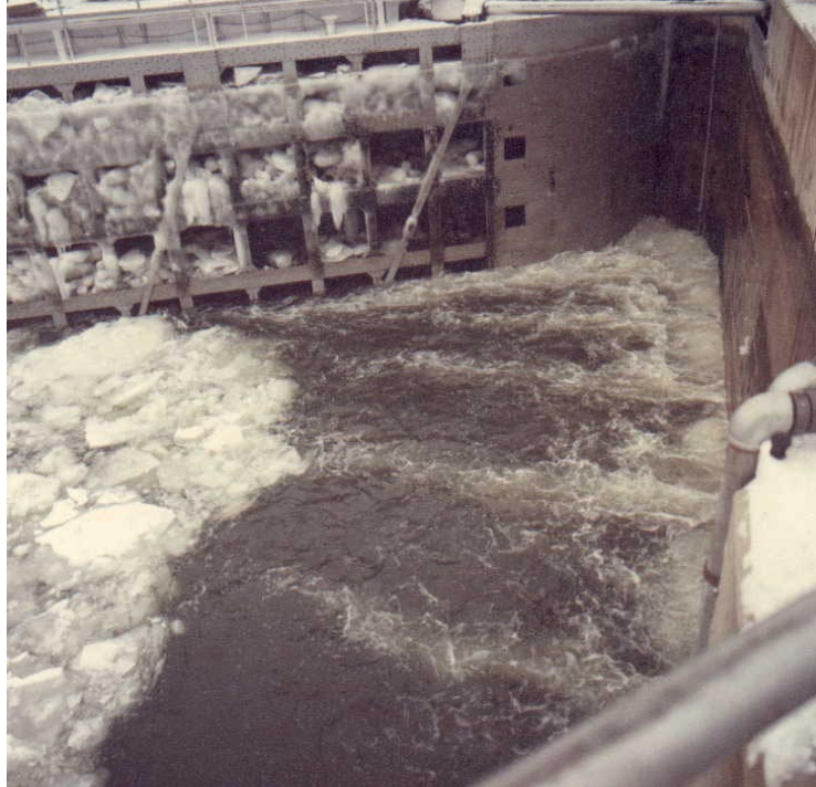
Figure 17. Gate recess flusher at Starved Rock Lock.
