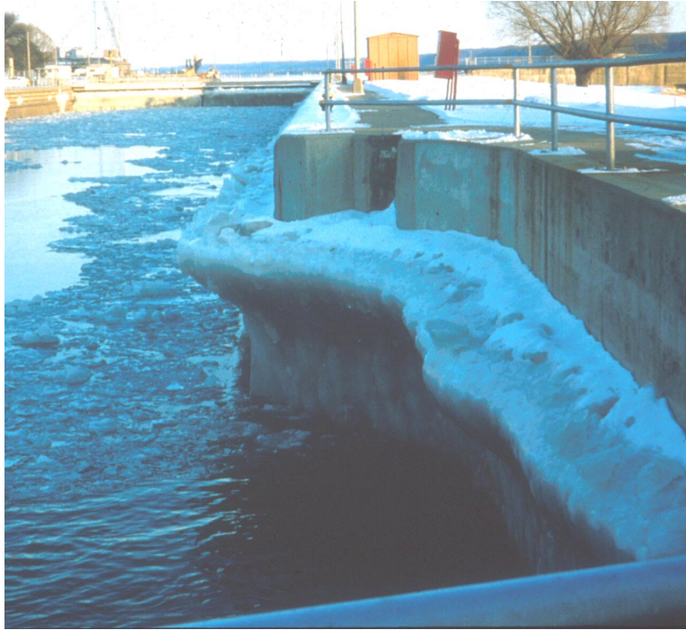
Figure 7. Ice collars in the gate recess and on the lock wall.
