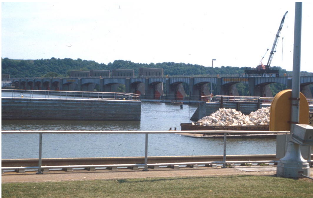
Figure 13. Drift pass in the river guardwall being widened at Lock and Dam 25 on the upper Mississippi.
