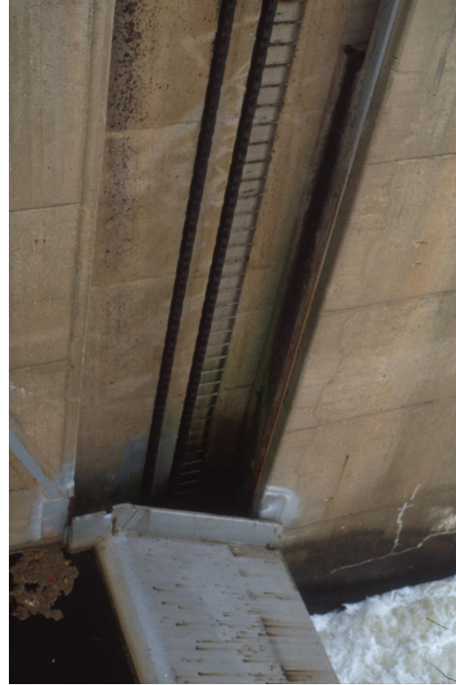
Figure 21. Direct lift gate at Montgomery Dam.
