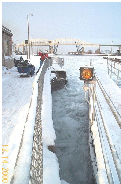
Figure 6. Clearing brash ice from the gate recess with a pike pole at the Soo Locks.
