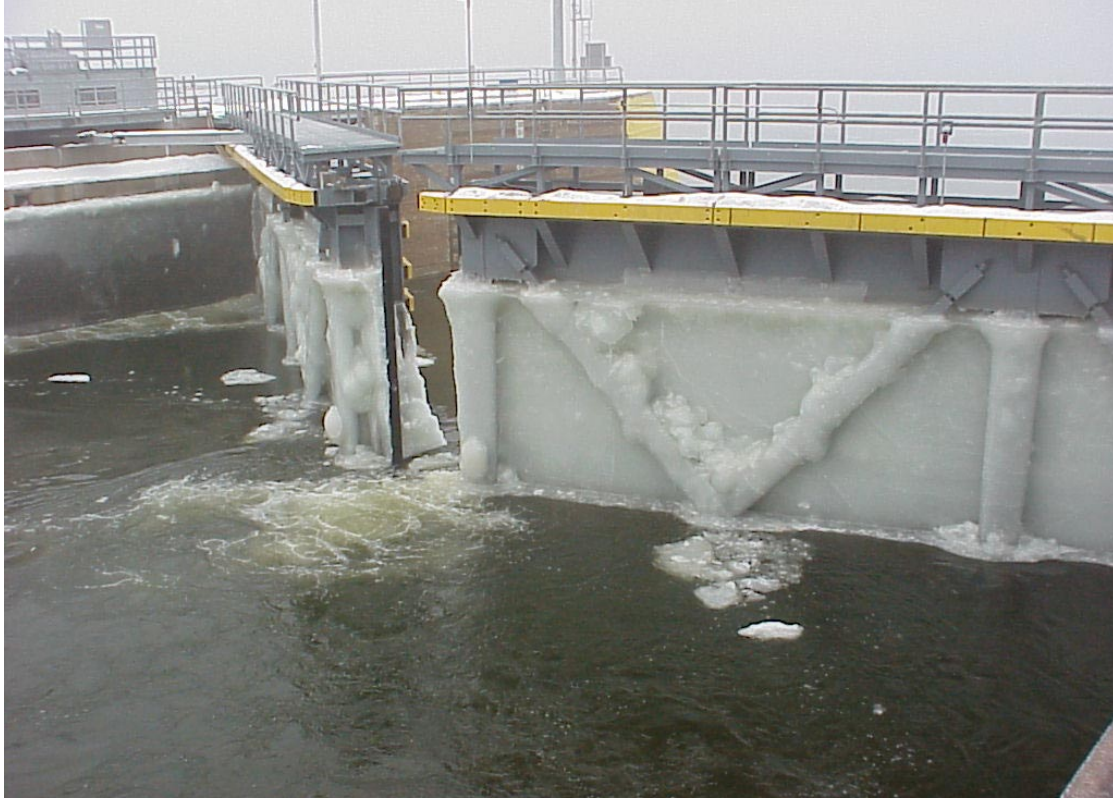
Figure 10. Miter at Lock 24 on the upper Mississippi with widely spaced structural members on the upstream side.
