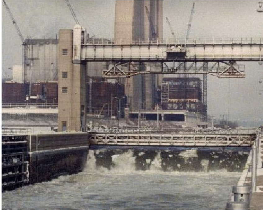
Figure 11. Skimming ice over emergency bulkheads at New Cumberland Lock on the Ohio River.
