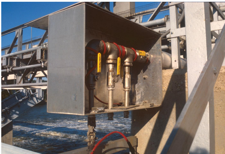
Figure 22. Steam manifold at Starved Rock Dam.
