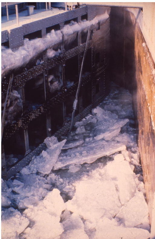
Figure 5. Brash ice in the miter gate recess.
