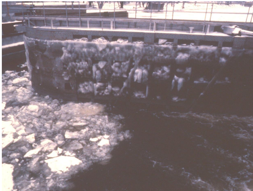
Figure 9. Icing of the miter gate trusswork.
