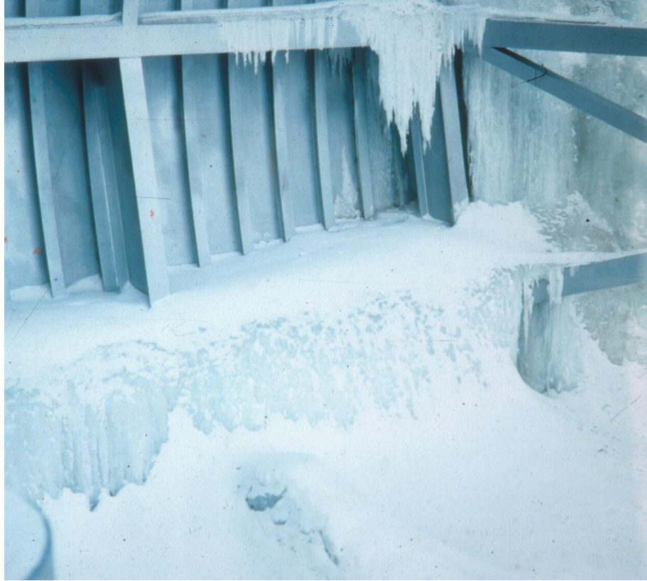
Figure 19. Iced-in tainter gate.
