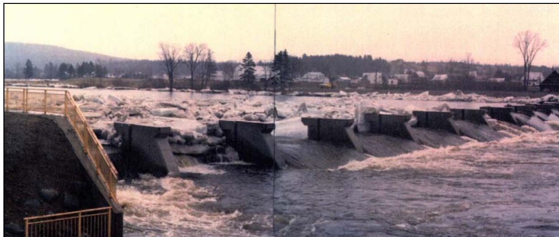
Figure 4. Weir-with-piers ice control structure on the Ste. Anne River at St. Raymond, Quebec.
