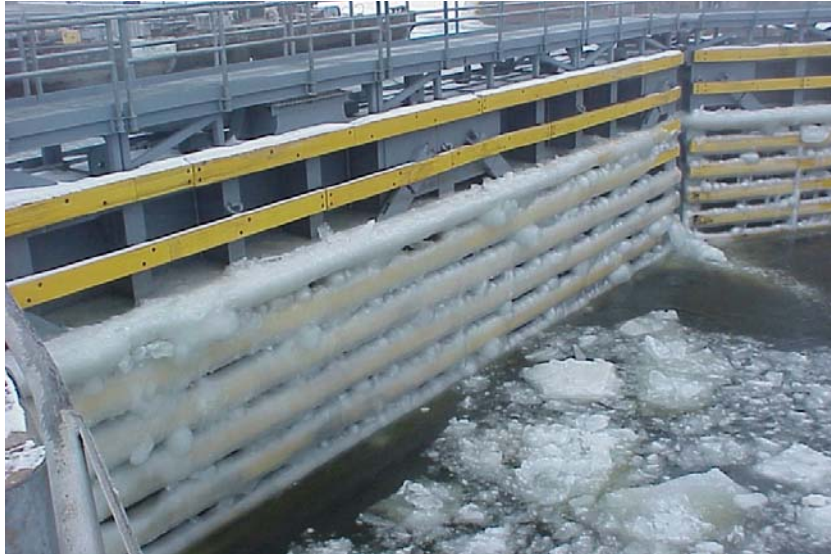
a. Miter gate with yellow, ice-covered rub rails, similar to gate where test piles were fielded.
