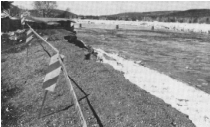
a. Bridge and road section destroyed.
