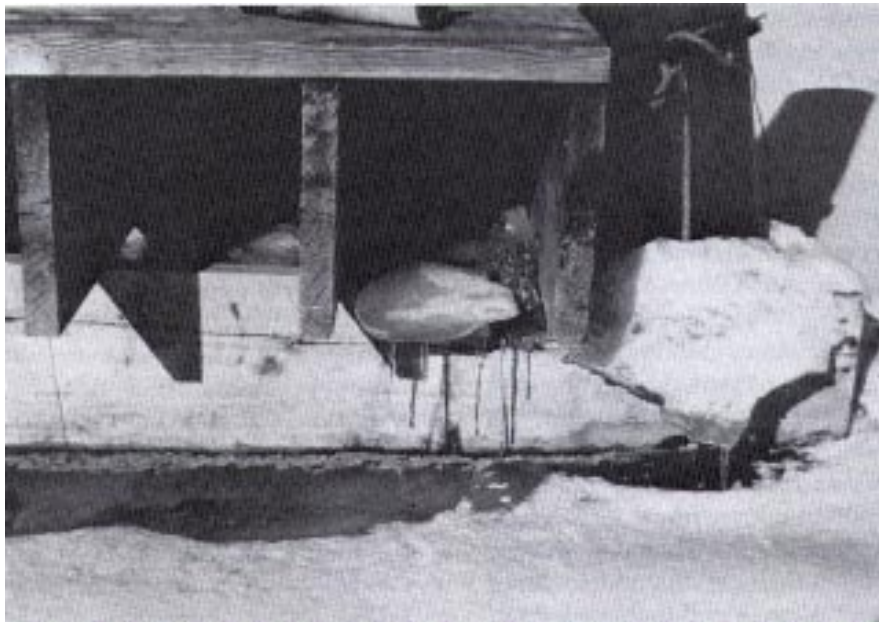
Figure 14. Horizontal member of dock in contact with the ice cover.
