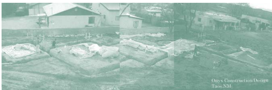
Onyx Construction, a local company, has provided much of the construction work for the casitas.
