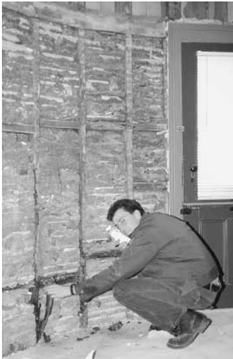
Peirce's former study during destructive investigation. Exhibit Specialist Paul Jaeger points to decaying exterior wall framing damaged over the years by moisture wicking through the riverstone veneer installed by Peirce in 1909.
