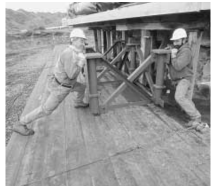
Jim Matyiko and Richie Meekins of Expert House Movers install temporary support system. Photo by Mike Booher.
