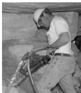
Mike Vakanti removes foundation stones before the lighthouse can be lifted from its present foundation. Photo by Mike Booher.
