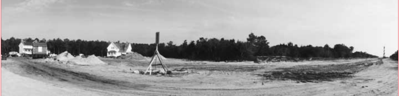
The move corridor. The lighthouse is at the original location on the far right. The keeper's quarters are positioned in their new site on the left. Photo by Mike Booher.
